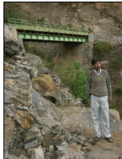
Fig. 2.10b: A portion of the link road to Chāyēen fell about 6 m
